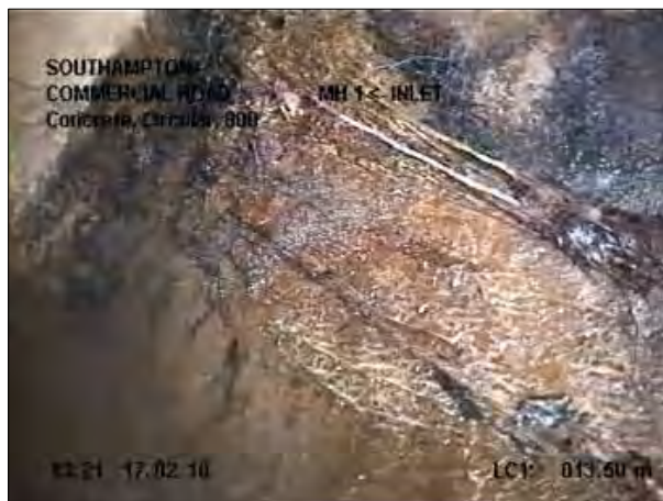
Photo: 15_13a, Tape No.: 1 13.5m, Mass Roots 10 % cross-sectional area loss
