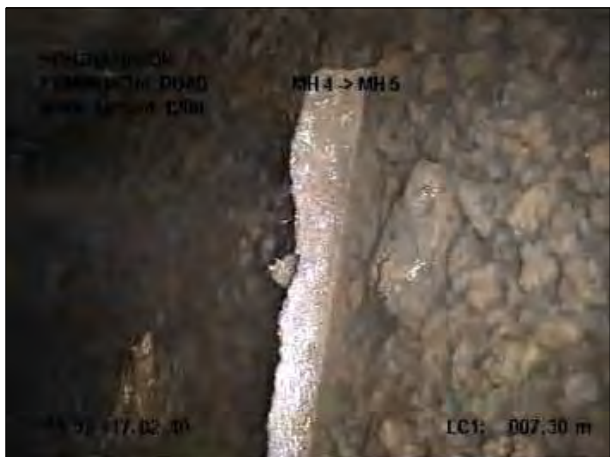
Photo: 62_6a, Tape No.: 1 7.3m, Obstruction, 30 % height/diameter loss
