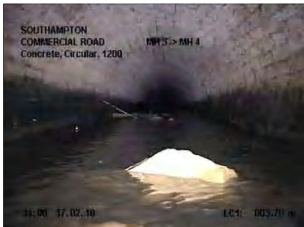
Photo: 47_7a, Tape No.: 1 3.7m, Obstruction, 30 % height/diameter loss
