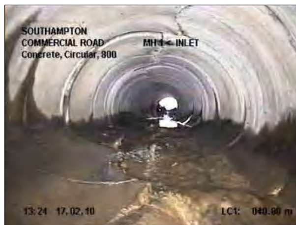
Photo: 21_18a, Tape No.: 1 40.8m, Sewer Broken, from 05 to 07 o'clock, Start
