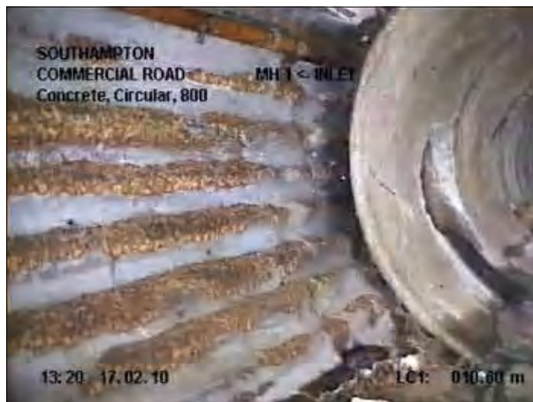
Photo: 11_9a, Tape No.: 1 10.6m, General Observation, Remark: REPAIR MADE
