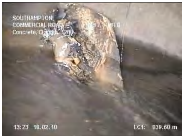
Photo: 94_10a, Tape No.: 1 39.6m, Obstruction, 30 % height/diameter loss
