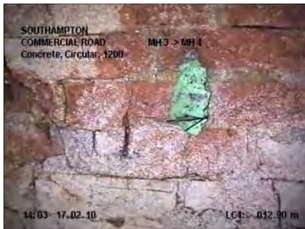
Photo: 49_9a, Tape No.: 1 12.9m, Hole in sewer from 01 to 02 o'clock
