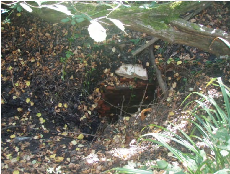
Figure 3. Small culvert entrance now blocked and in bad state of repair (culvert requirement no longer obvious).
