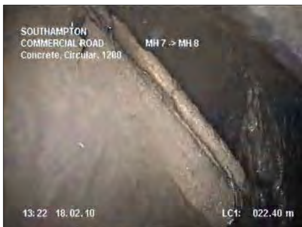
Photo: 92_8a, Tape No.: 1 22.4m, Obstruction, 20 % height/diameter loss
