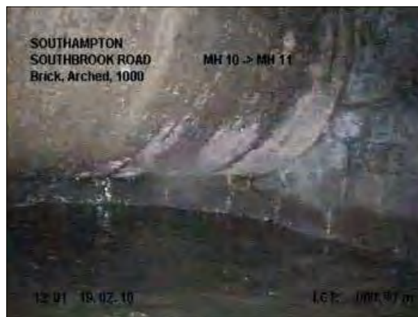
Photo: 131_9a, Tape No.: 1 0.9m, General Condition photograph, Remark: SERVICE PIPE PASSING THROUGH
