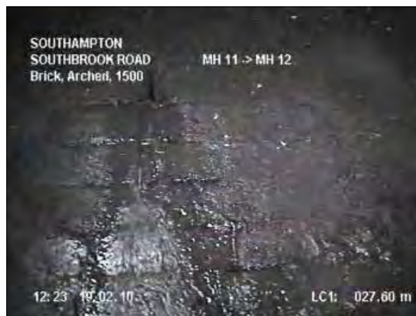
Photo: 158_7a, Tape No.: 1 27.6m, Infiltration Gushing from 08 to 10 o'clock
