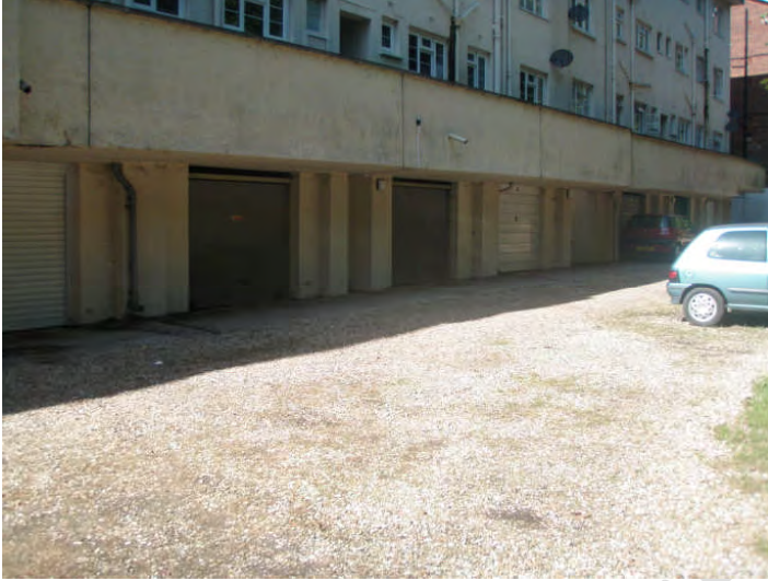
Figure 9. Main flow of brook is through a culvert under concrete hard standing.
