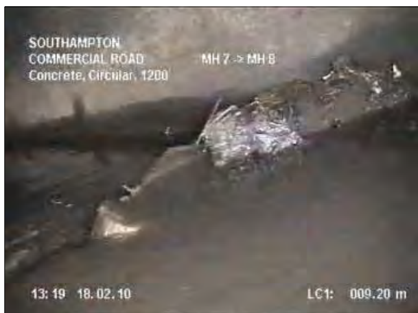
Photo: 88_4a, Tape No.: 1 9.2m, Obstruction, 30 % height/diameter loss
