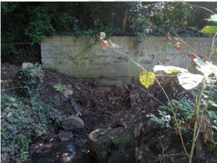
Figure 15. Blocked trash screen with primarily with Japanese Knotweed debris.
