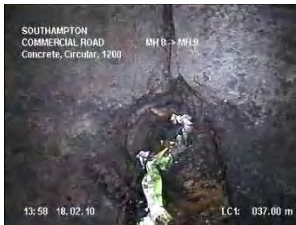
Photo: 107_8a, Tape No.: 1 37m, Connection defective, at 02 o'clock, dia 150 mm
