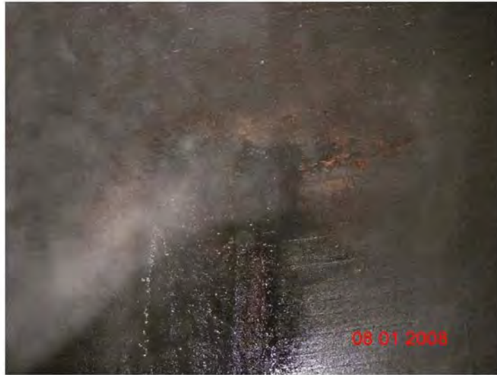
Photograph No 3 Water seepage at -5000mm to 0mm
