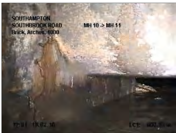
Photo: 131_9b, Tape No.: 1 0.9m, General Condition photograph, Remark: SERVICE PIPE PASSING THROUGH
