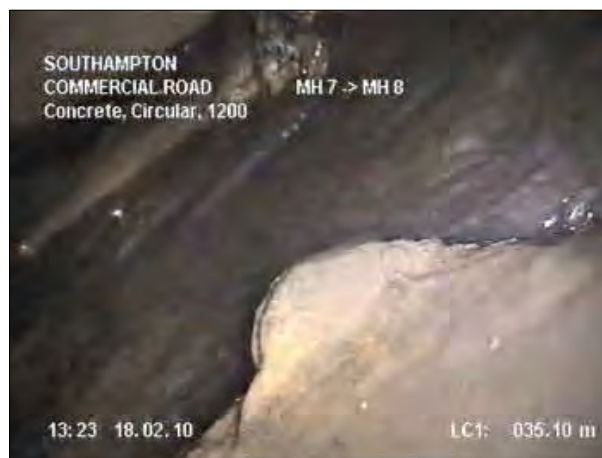
Photo: 93_9a, Tape No.: 1 35.1m, Obstruction, 30 % height/diameter loss
