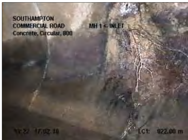
Photo: 16_14a, Tape No.: 1 22m, Mass Roots 10 % cross-sectional area loss
