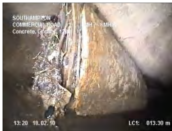
Photo: 89_5a, Tape No.: 1 13.3m, General Observation, Remark: WOODEN PLANKS
